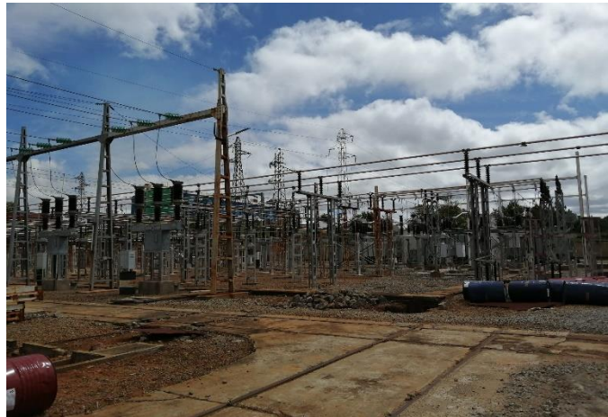
Picture 4. Main production site of the JIRAMA national company.
